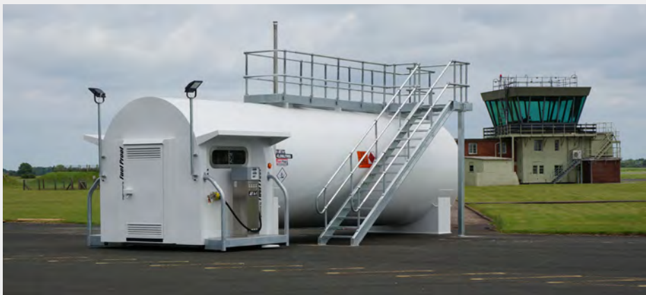
42,000L PREMIUM BULK JET A-1 TANK MANUFACTURED AND INSTALLED AT LEEDS EAST AIRPORT
