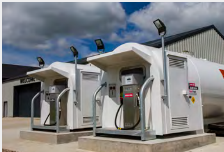
15,000 LITRE JET A-1 AND AVGAS BULK TANKS
